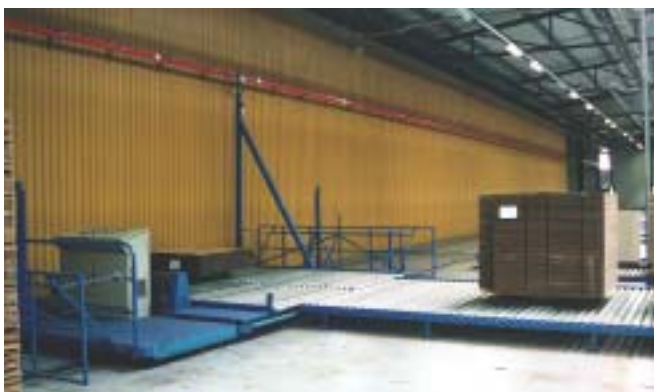
Conductor housing, type RN7 for feed and control of a traverse car in a carton processing plant.
